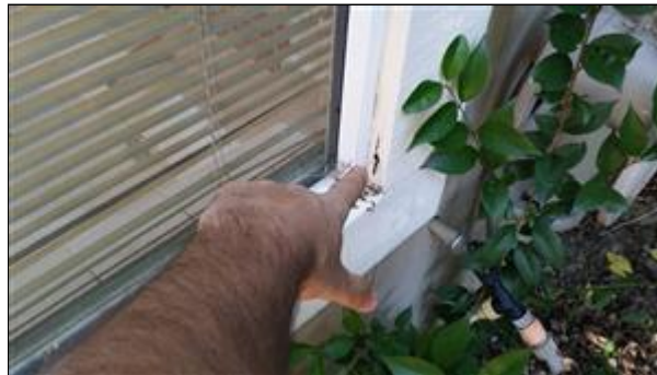
2.1 Picture 2 Wood Rot (Rear Living Room)
