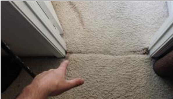
4.2 Picture 3 Damage (Master Bathroom)
