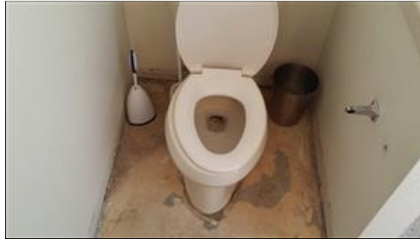
4.2 Picture 5 Damage (Master Bathroom)
