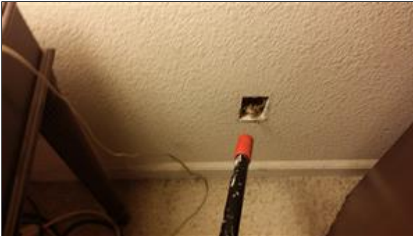
7.2 Picture 3 Missing Receptical (Office)
