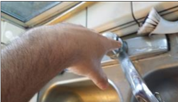
6.1 Picture 4 Leak at Handle (Kitchen Sink)
