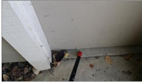
2.1 Picture 1 Delaminating (Left Side Garage Door)
