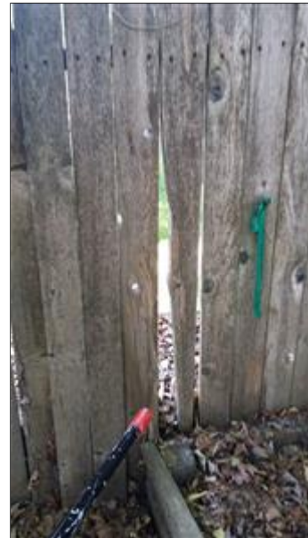
2.6 Picture 3 Broken Picket (Left Side)
