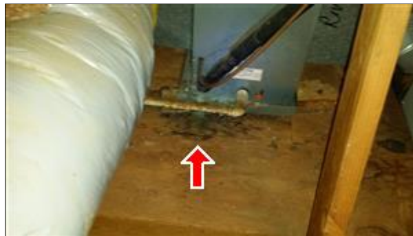
8.0 Picture 3 Water Damage (Attic)
