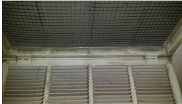
8.0 Picture 1 Dirty Return Filter (Hallway)
