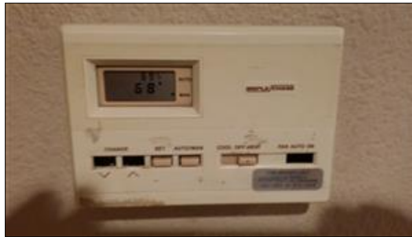
8.7 Picture 2 Damaged Thermostat (Hallway)
