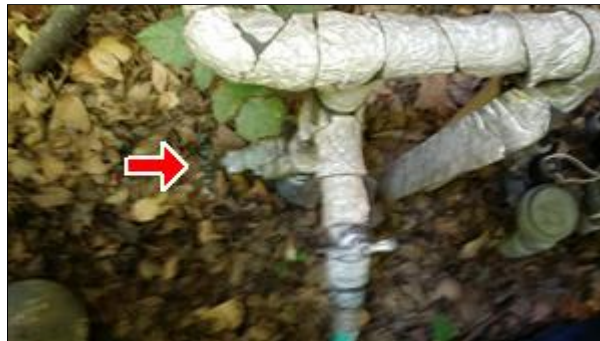
6.3 Picture 1 Main Water Shut Off (Front Entry)
