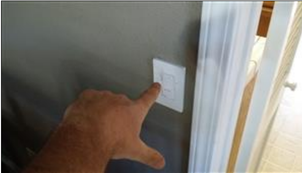
7.2 Picture 2 Damaged Switch (Dining Room)
