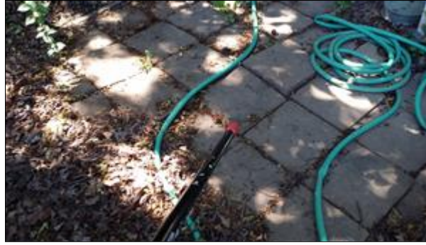
2.3 Picture 1 Uneven Pavers (Rear Left)
