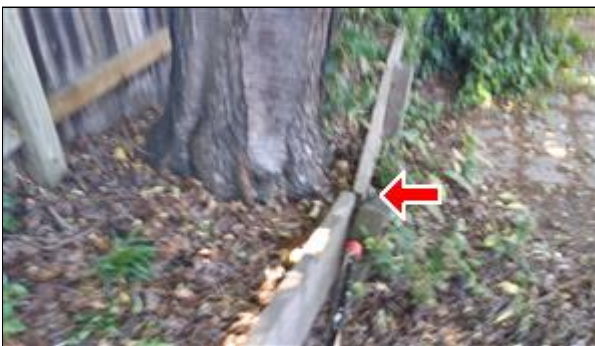
2.4 Picture 2 Damaged Retaining Wall
