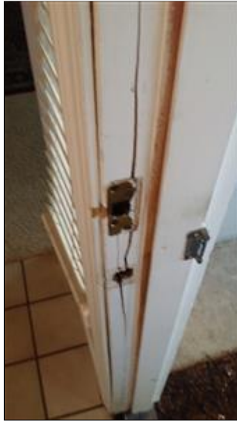
4.4 Picture 1 Damaged Front Door And Jamb
