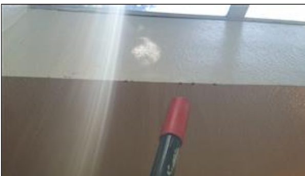
4.5 Picture 2 Stains (Kitchen SkyLight)
