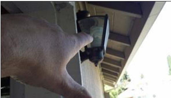
7.2 Picture 4 Dead Bulb (Left Side Garage)
