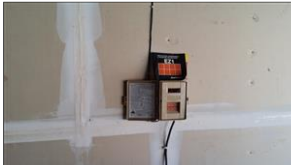
6.6 Picture 3 Front Irrigation Timer (Garage)
