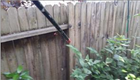
2.6 Picture 10 Rotted Fence Post (Right Side)
