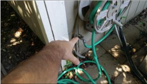
6.1 Picture 1 No Water Flow (Left Rear)
