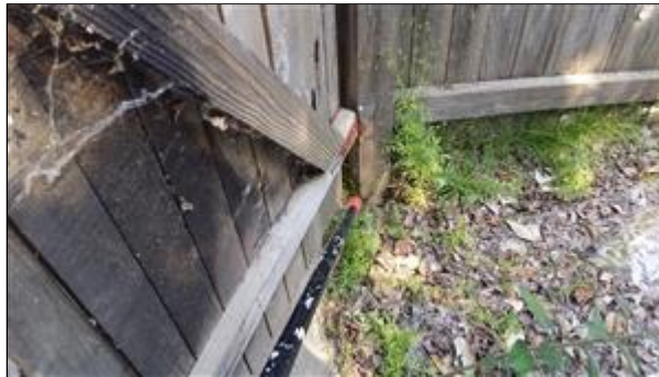
2.6 Picture 2 Rotted Gate Post (Left Front Gate)
