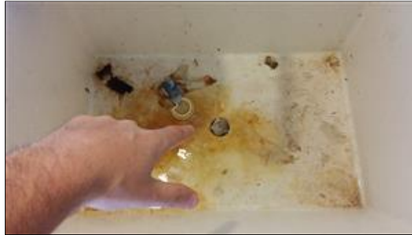
6.1 Picture 5 Slow Drain (Garage)
