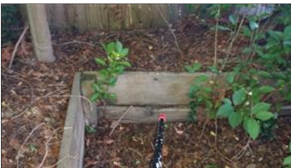
2.4 Picture 3 Damaged Retaining Wall (Rear)
