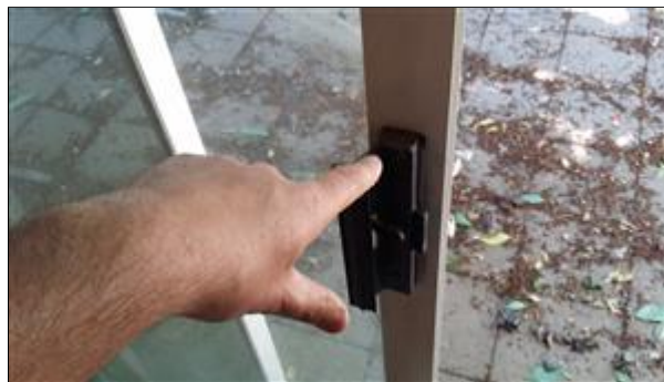
4.4 Picture 3 Loose Fixture (Master Bedroom)
