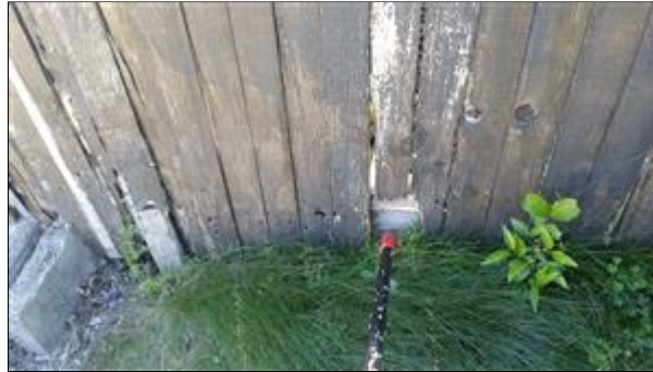
2.6 Picture 1 Damaged Picket (Near Left Side Gate)
