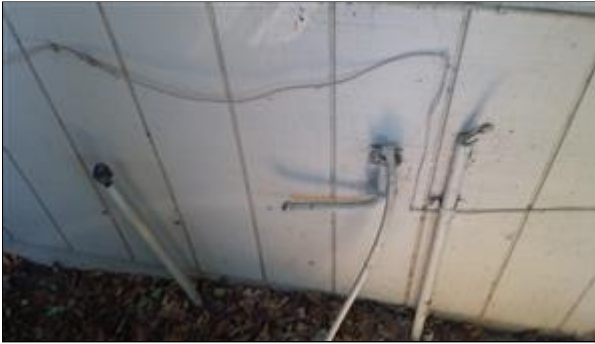
7.2 Picture 1 Abandon Wiring (Right Rear)
