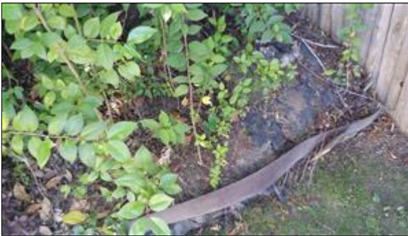
2.4 Picture 1 Deteriorated Retaining Wall ( Front Right)
