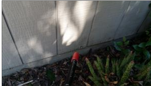
2.0 Picture 1 Rotted Siding (Rear Master Bathroom)
