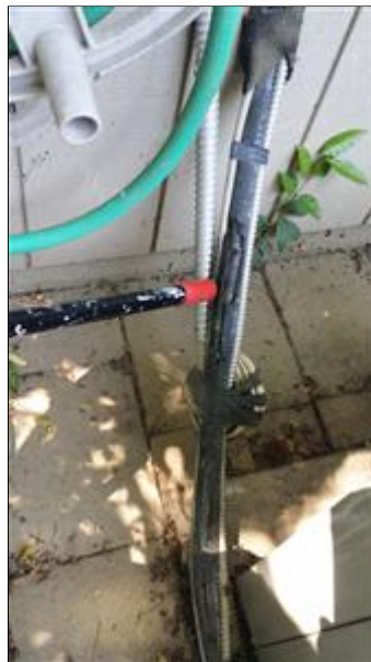
8.6 Picture 1 Deteriorated Suction Line Insolation
