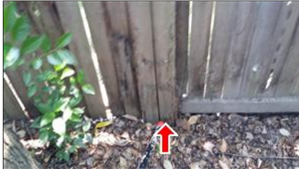
2.6 Picture 6 Rotted Fence Post (Left Side)
