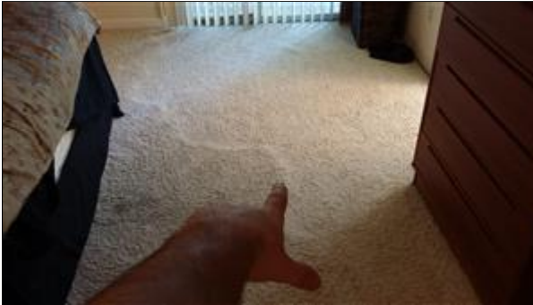
4.2 Picture 2 Damaged (Master Bedroom)
