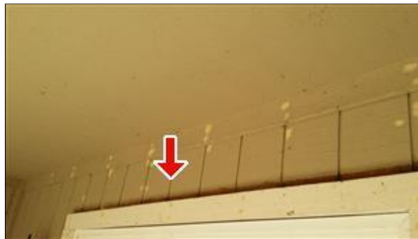
2.1 Picture 3 Unfinished Trim and Siding
