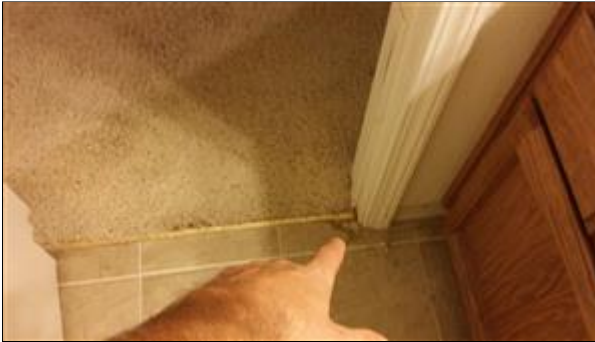
4.2 Picture 1 Damage (Bathroom & Hallway)
