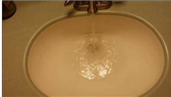
6.1 Picture 6 Slow Drain (Right Bathroom Sink)
