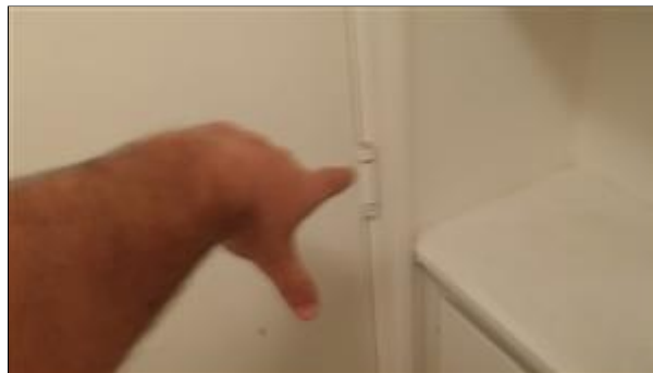
3.4 Picture 1 Dysfunctional Hinge (Garage Door)
