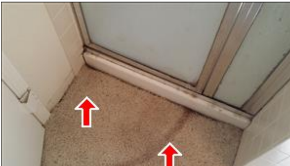
4.2 Picture 4 damage (Master Bathroom)
