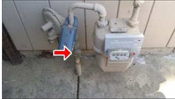
6.5 Picture 1 Main Gas Shut Off
