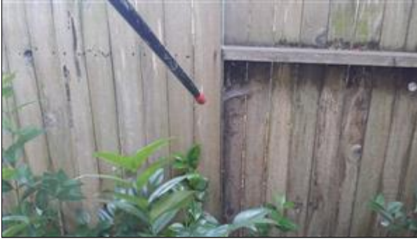
2.6 Picture 9 Rotted Fence Post (Right Side)
